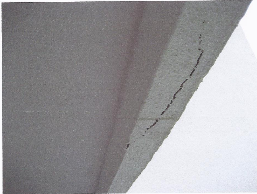
View of typical concrete spall in turned-down perimeter beam
