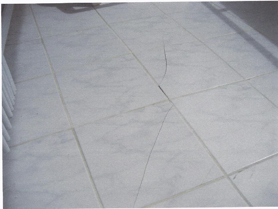
Example of probable concrete spalling under cracked tile on balcony
