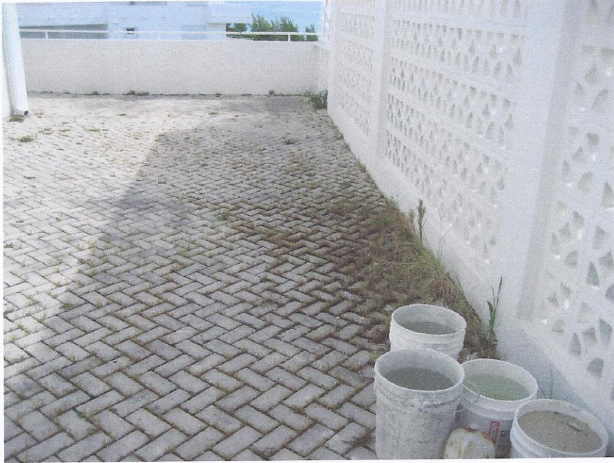
View of Pavers on Penthouse balconies-poor protection for structure
