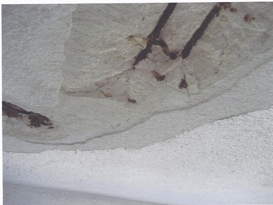
View of exposed concrete spall and rebar corrosion on walkway ceiling
