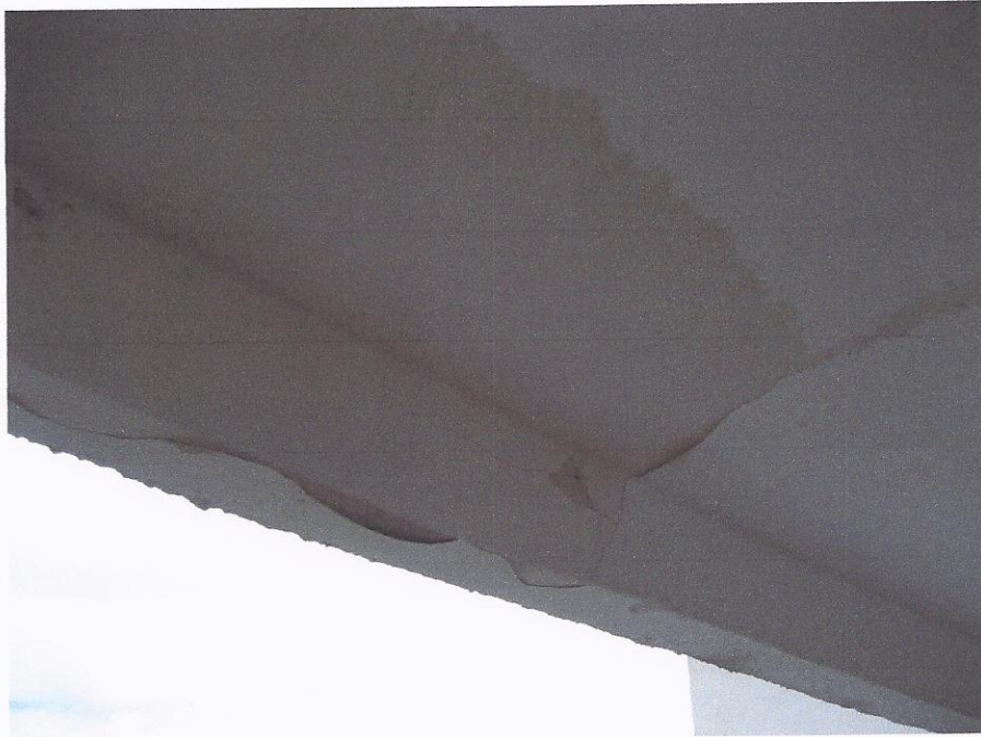
View of improper heavy elastomeric paint applied to walkway ceiling
