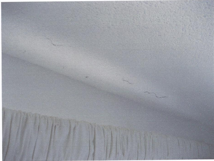
View of interior concrete spalling at ceiling near balcony sliding glass door
