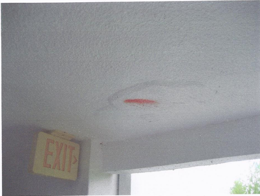
View of unexcavated ceiling spall
