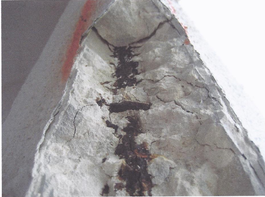
Example of spalled concrete at vertical support column
