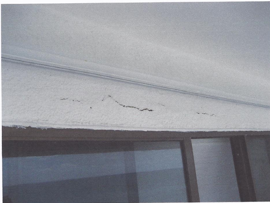
Example of spalled header beam above sliding door
