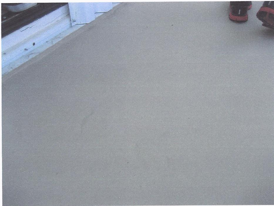
Example of unexcavated floor spalls
