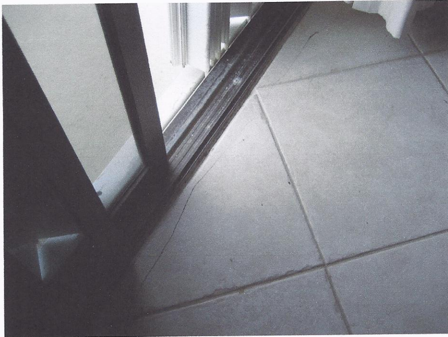
Example of probable interior spalling under cracked tile
