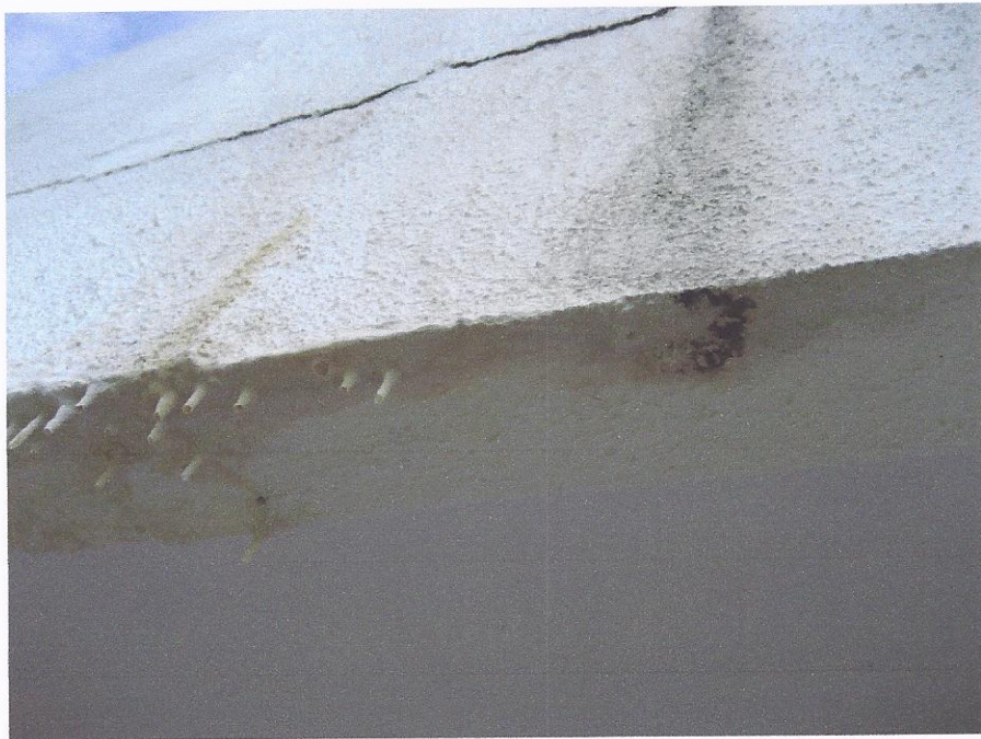
View of leaking evidence at Walkway knee wall edges
