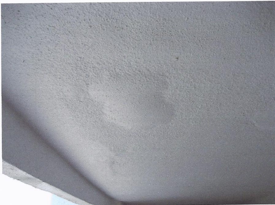
View of paint bubble in ceiling due to water intrusion trapped by elastomeric coating
