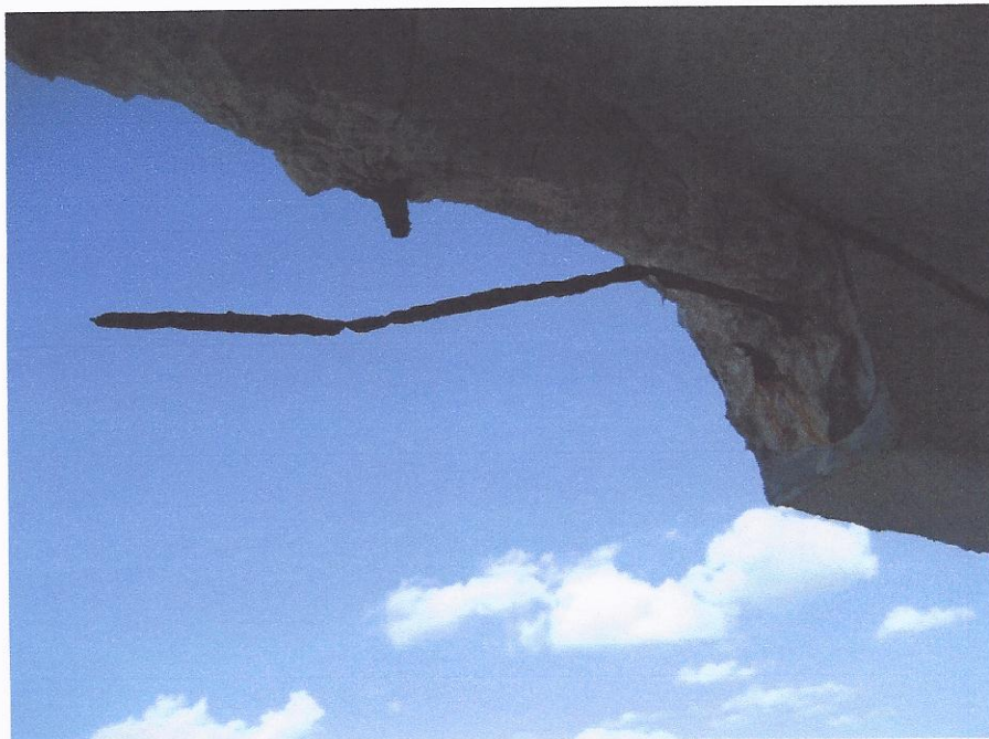
View of exposed reinforcing steel corrosion in turned-down perimeter beam Note-loss of cross sectional area of steel reinforcement due to corrosion activity
