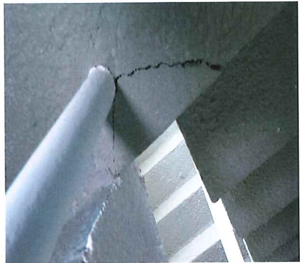
Photo #2 - illustrating moderate to severe concrete crack defects within the western stairwell.
