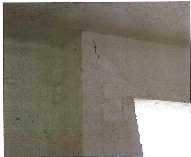
Photo #4 - illustrating moderate, concrete crack defects at the eighth (8th) floor near room #82.
