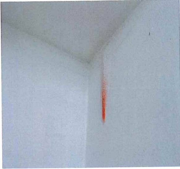
Photo #9 illustrating moderate concrete crack defects at the eastern stairwell CMU walls.
