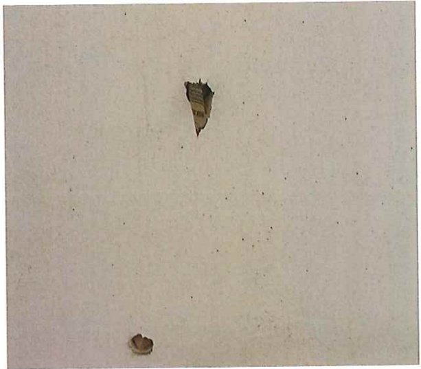
Photo #10 illustrating moderate concrete crack defects at the ceiling of the south western ground floor breeze-way area.
