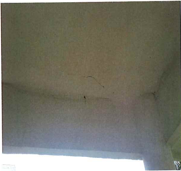
Photo #11 illustrating moderate, concrete crack defects at the concrete ceiling of the southern breezeway area.
