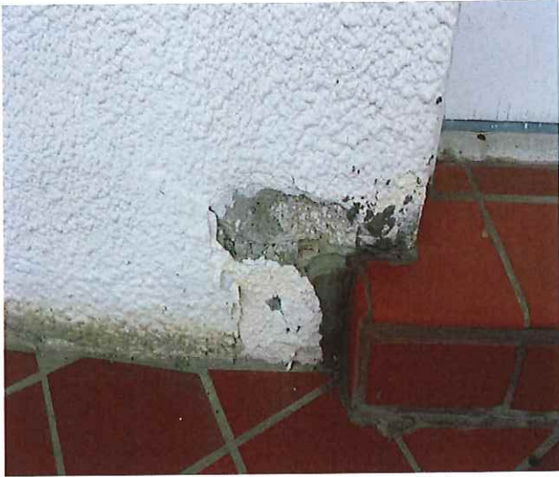
Photo #5 illustrating a moderate concrete crack defect at the base of the CMU wall within the walkway area.
