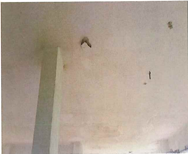
Photo #3 - illustrating severe, concrete crack defects within the ceiling at south-west ground floor ceiling areas exposed to the elements at the open "Breeze-way" areas.
