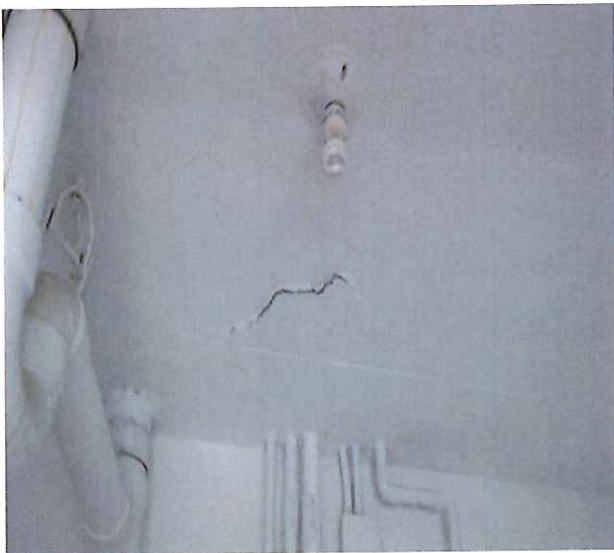
Photo #7 illustrating severe concrete crack defects within the Laundry room at the Sixth floor.
