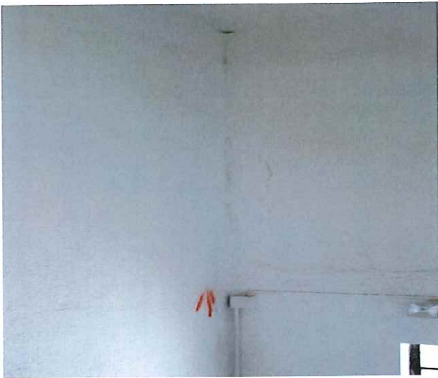
Photo #1 - illustrating moderate concrete crack defects within the eastern stairwell.
