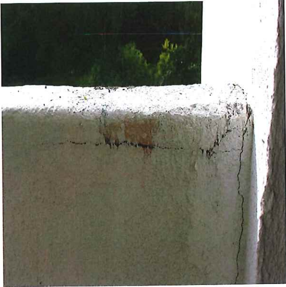
Photo#13 illustrating moderate, concrete crack defects at the CMU balcony rail.
