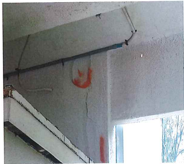
Photo #16 illustrating severe concrete crack defects at the reinforced concrete columns supporting the first level concrete beams at the south western breezeway area.
