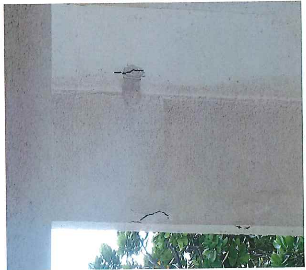
Photo #12 illustrating moderate concrete crack defects at the reinforced concrete beam supporting the second (2 nd ) Floor concrete floor slab at the south western ground floor breezeway area.
