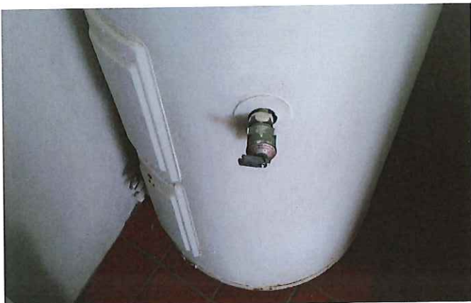
Photo #1- Illustrating that the water heater relief valves require a discharge pipe.
