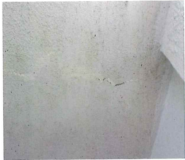
Photo #6 illustrating moderate concrete crack defects within the ceiling of the walkway.
