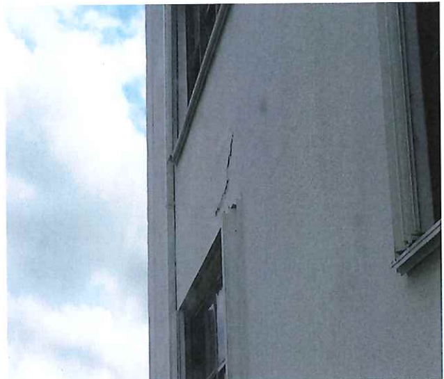
Photo #8 illustrating severe concrete crack at the exterior CMU wall at the south-east section.
